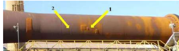
Figure 5 – Detail of Figure 1 showing the kiln shell with welded repair patches (e.g., arrow 1), and a repair consisting of a single weld bead (arrow 2).
