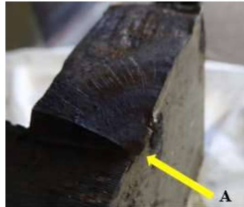
b) Detail of the crack propagation, starting at corner. Figure 8 – Crack surface of one of the broken eyebars.
