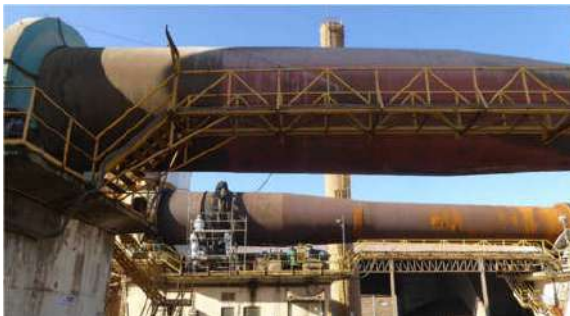
Figure 1 – Partial view of the kiln that suffered the failures, in the background. In the foreground, another kiln decommissioned since 2011.
