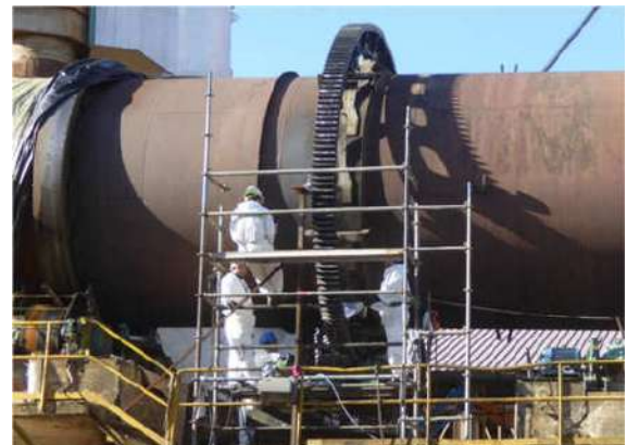
Figure 6 – Spring plates. a) Zoom of Figure 1, showing the toothed crown and spring plates (identified with arrows), undergoing repair/assembly work by technical staff.
